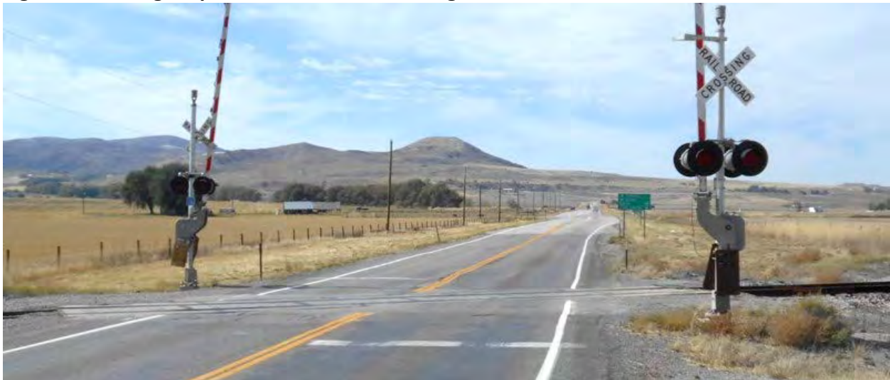
Figure 29: Fading Stop Lines at Railroad Crossing East of S.R. 23
